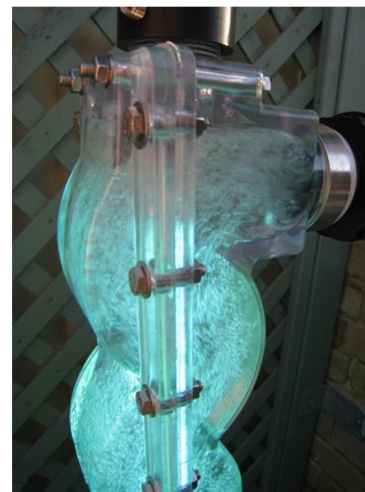
Combination UV & Ozone (Advanced Oxidation)
